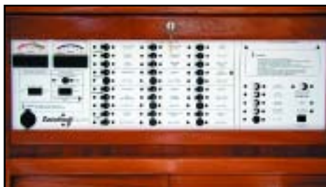
Complete electrical panel with provision for additions and options that may be added later.
